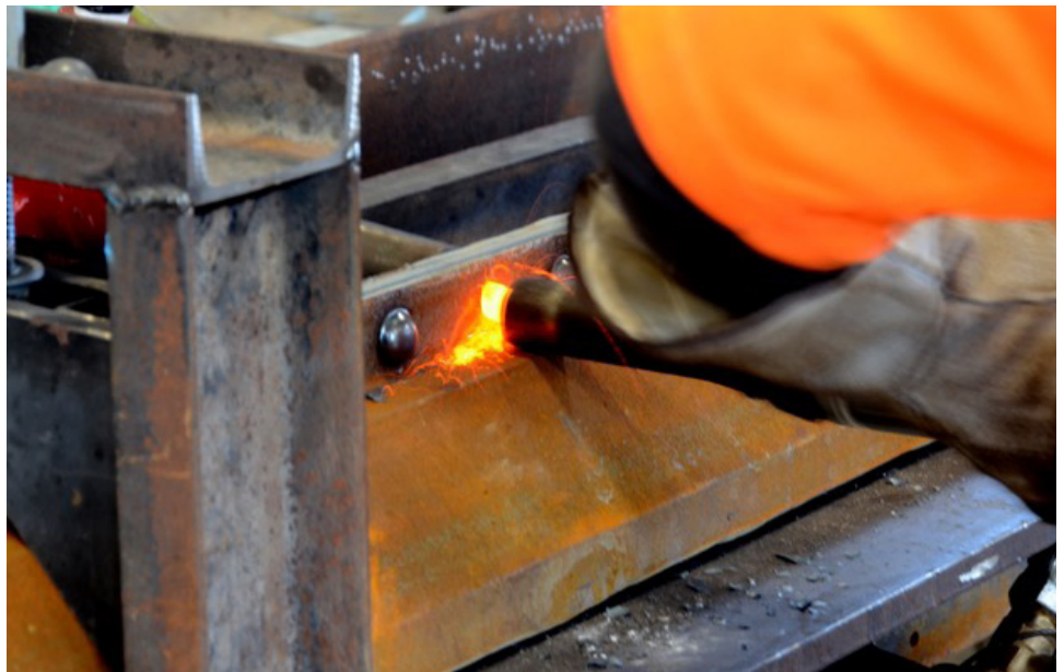
Hot riveting work on the Blackfriars Bridge. (Photograph courtesy of City of London, photographer MJ Idzerda)
